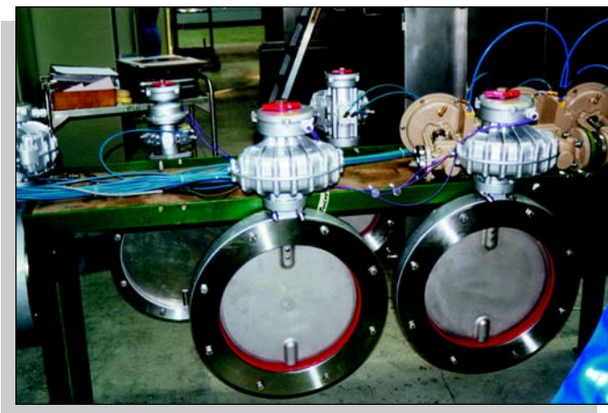
Figure 5. Simulated air handling unit at an FAT.
