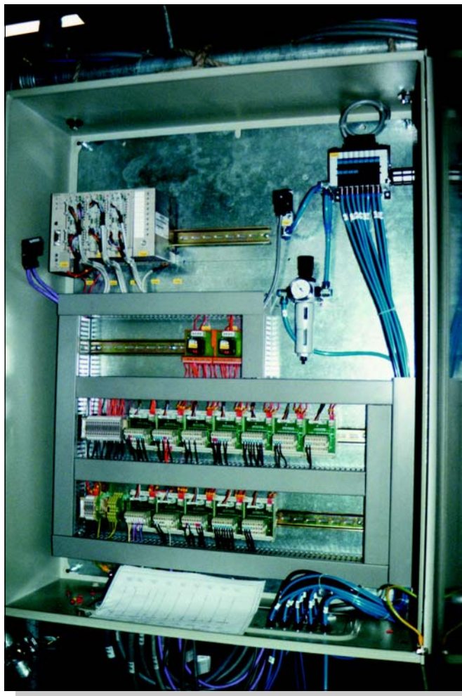
Figure 3. Electrical hardware check.
